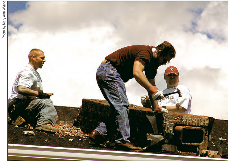
Construction workers repair the roof and chimney of St. Elizabeth's Pregnancy and Adoption Services' residential building on May 31, a day after a tornado caused structural damage to the archdiocesan property. St. Elizabeth's ministers to young women who are experiencing crisis pregnancies and to their families.
