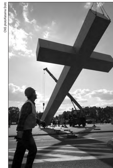
Workers erect a large wooden cross on May 10 on the altar that will be used for Pope Benedict XVI's Mass in Pilsudski Square in Warsaw. The pope will visit Poland on May 25-28.
