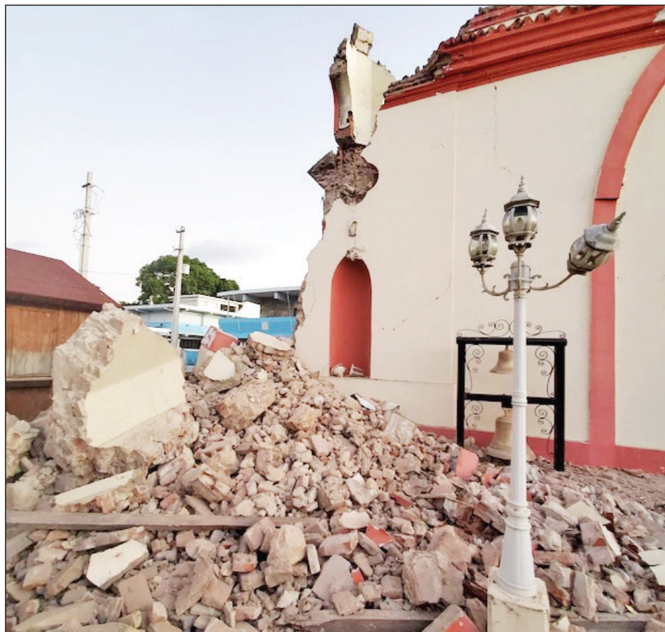
The destroyed Immaculate Conception Church in Guayanill, Puerto Rico, is seen on Jan. 7 following recent earthquakes in Puerto Rico. A magnitude 6.4 quake rattled Puerto Rico before dawn, killing at least two people and setting people on edge. (CNS photo/courtesy Diocese of Ponce)
